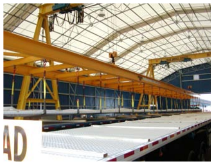
This beam with a very long span is used with two cranes.
